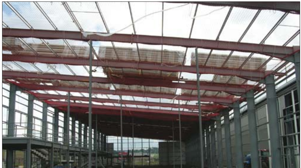
Figure 7 Safety nets installed prior to sheeting. Note that the net is fixed as close to the underside of the roof as possible to minimise the extent of any fall
