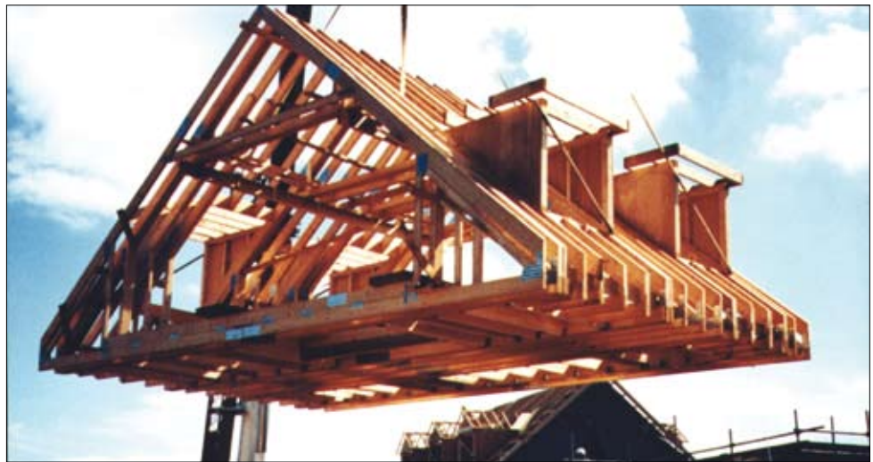
Figure 6 Roof truss built on the ground and lifted into position, avoiding the need to work over open joisting later on
