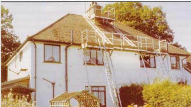
Figure 3 Proprietary access system for roof work
